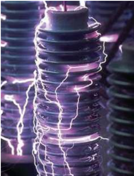
Electric breakdown of and power insulator
